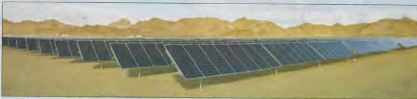
Energy focus... Namibia is endowed with excellent untapped renewable resources more than sufficient to meet domestic energy needs.
